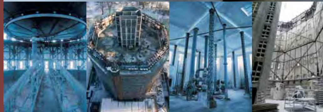
Spiral staircase to Cave Bar, 1: View into the lower water tank, 2nd.1.: Newly constructed concrete core finished to the 19th floor, 2nd.r.: Pumps and valves of the original water installation, r.: Building in the new ceilings into the historic facade Wendeltreppe zur Cave Bar, 1: Blick in den unteren Wassertank, 2. v. l.: neuer Betoneinbau bis zur 19. Etage fertiggestellt, 2. v. r.: Pumpen und Schieber der Original-Wasserinstallation, r.: Einbau der neuen Etagendecken in die historische Fassade
